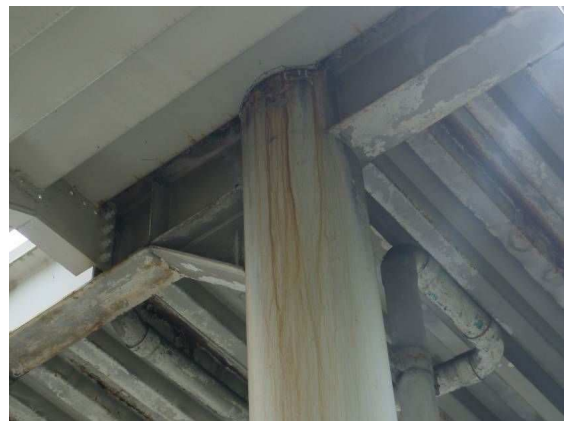
柱鋼管の塗膜劣化, 腐食
